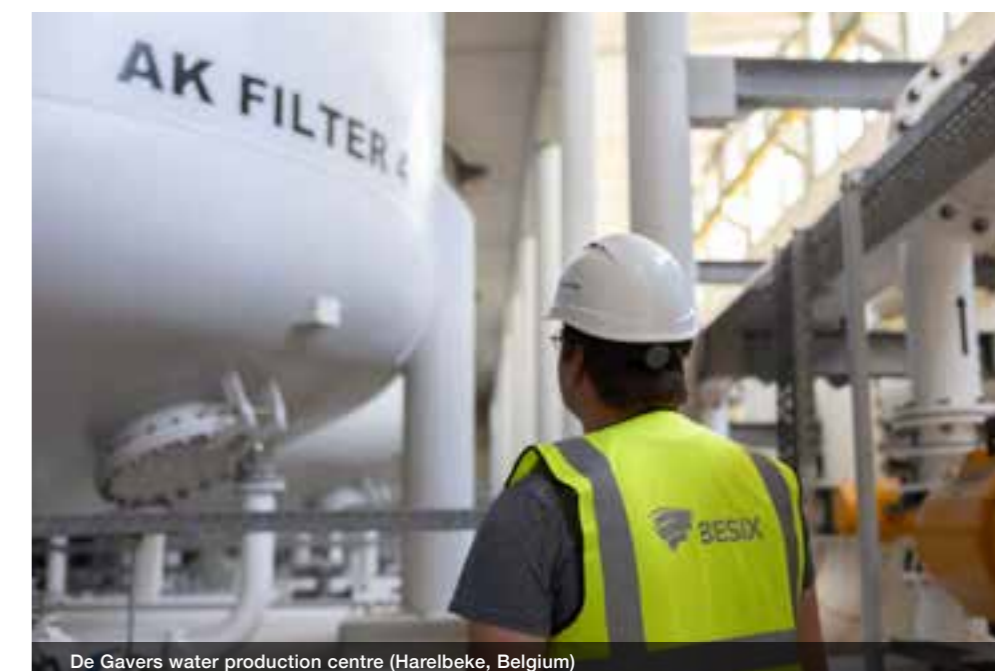
De Gavers water production centre (Harelbeke, Belgium)
